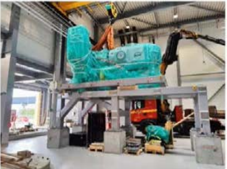
MAN Compressor @ site in Esbjerg
