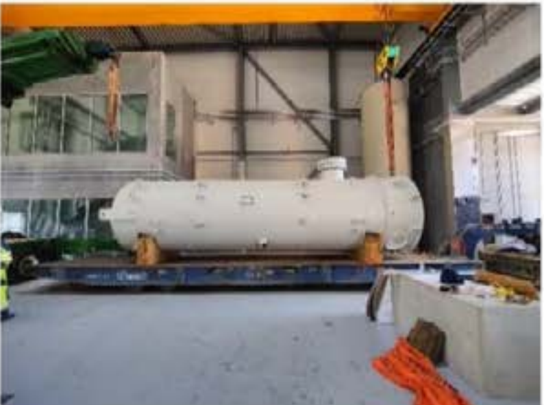
CO 2 storage tank
